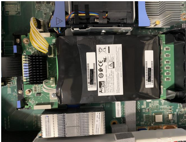
Figure 22. Battery backup unit
