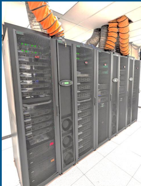
GPU Server Rack
