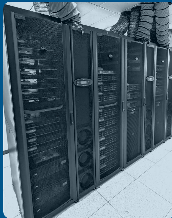
Our on-prem GPU server rack
